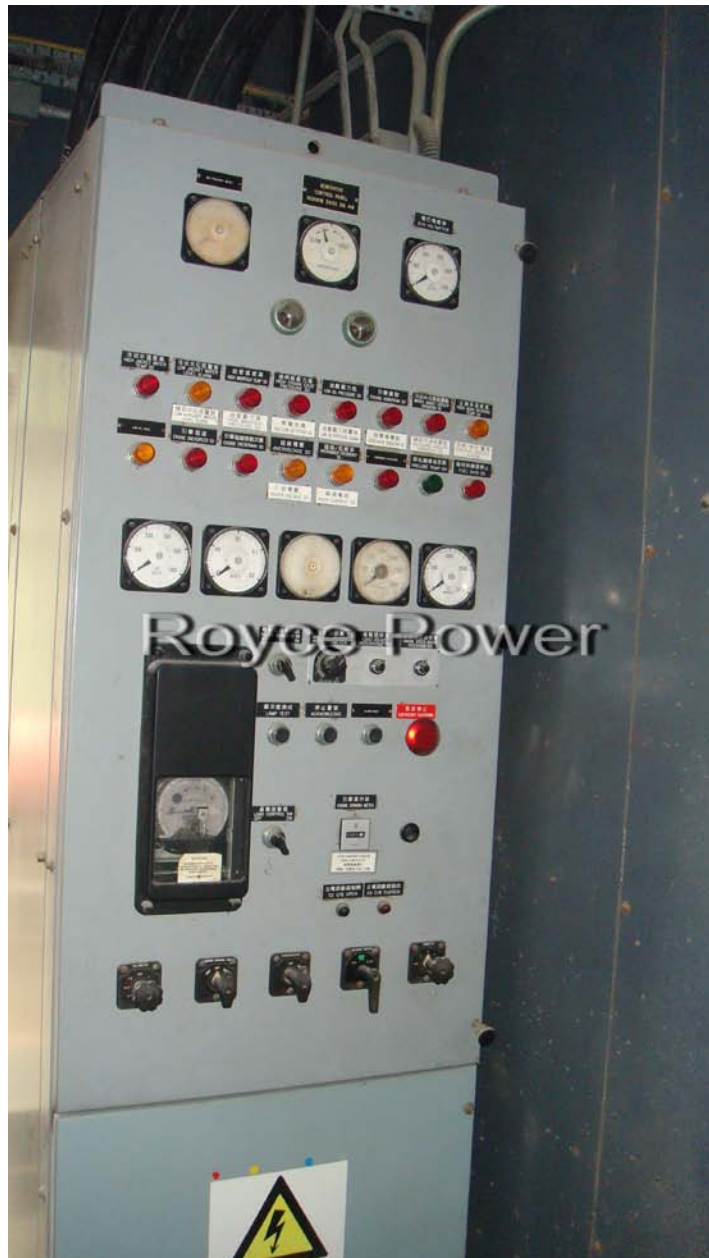
Generator Control Panel
